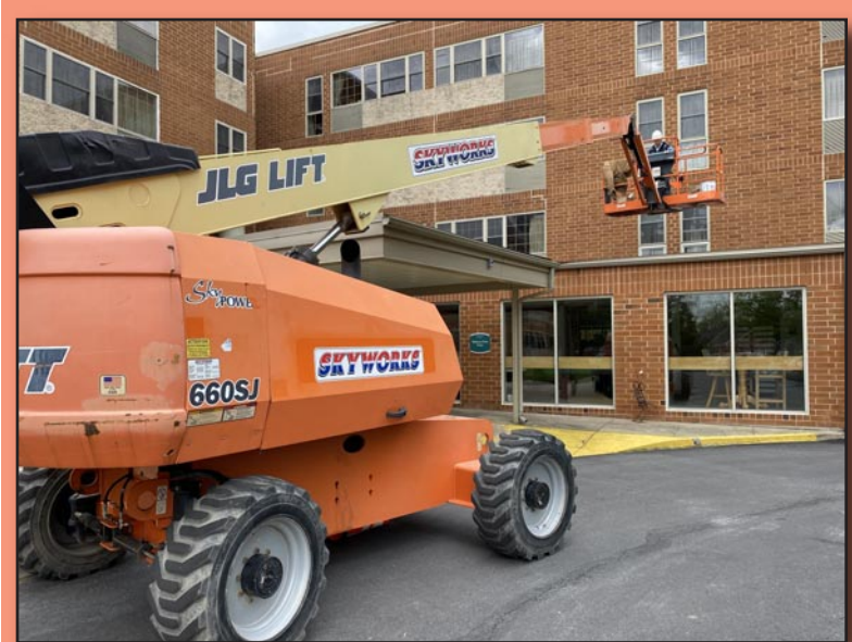
The Central PA Chamber always enjoys seeing members working together. Recently, Skyworks Equipment Rental provided a 65-foot straight boom lift to XW Construction for a job at the Warrior Run Manor. It was used to help with caulking and weatherizing windows. Pictured in the basket is David Zook of Zook's Enterprises, who also works with XW Construction. Learn more about these members at centralpachamber.com/membership-directory .
